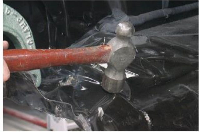
B Hammer blows with pulling traction will help relieve stress and aid in pulling other panels into alignment.
