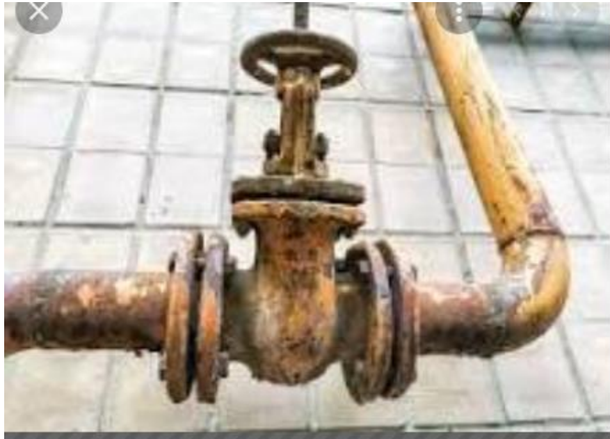
Fig 2.9 Deteriorating cast iron pipe
