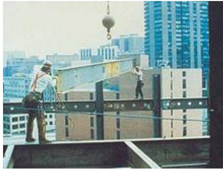
At-risk workers without appropriate safety equipment
